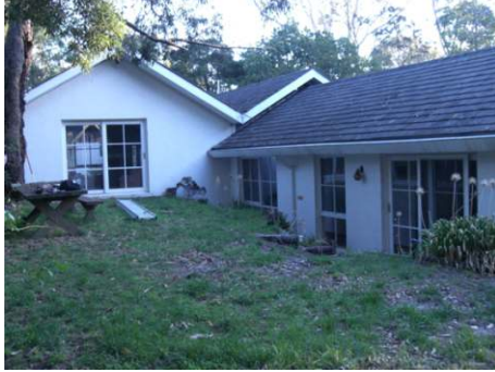
Existing level problems and poor condition of retaining wall
